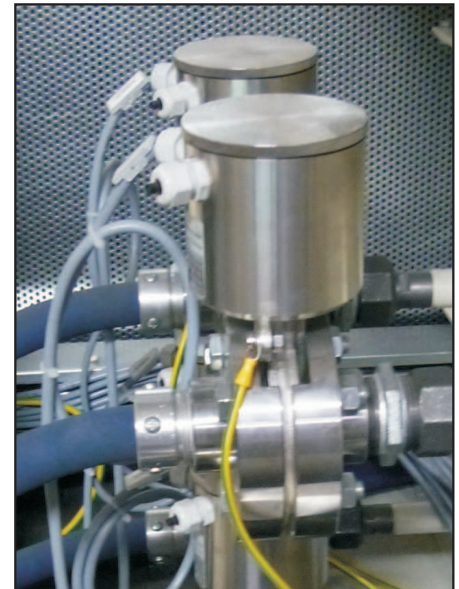
Installation at a shotblasting system
